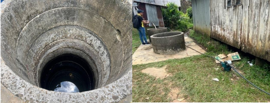
Figure 8.3. The condition of the water in the well is questionable and do not have proper covers to prevent contamination
